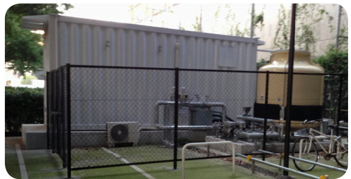
Fig. 3. Exterior view of TSUBAME-KFC: evaporative cooling tower right next to the 20-foot module for complete lights-out operation and low waterpump power
