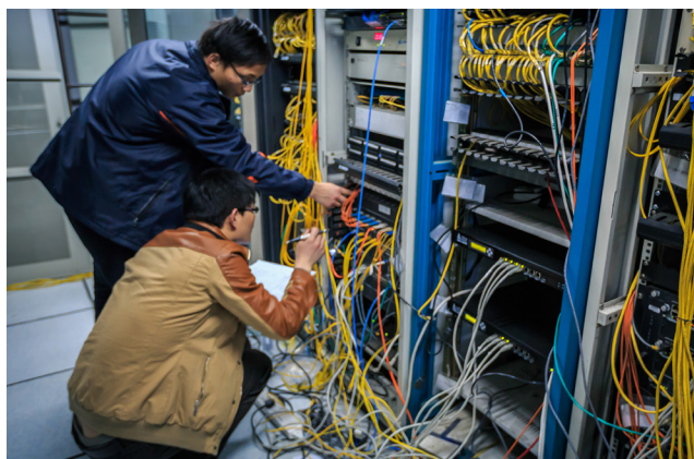
Air-cooled data centers do not provide for technician comfort or ICT workspace.
