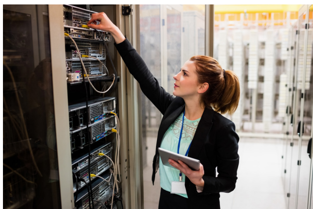
Air-cooled vertical rack height can make access to some ICT equipment difficult.
