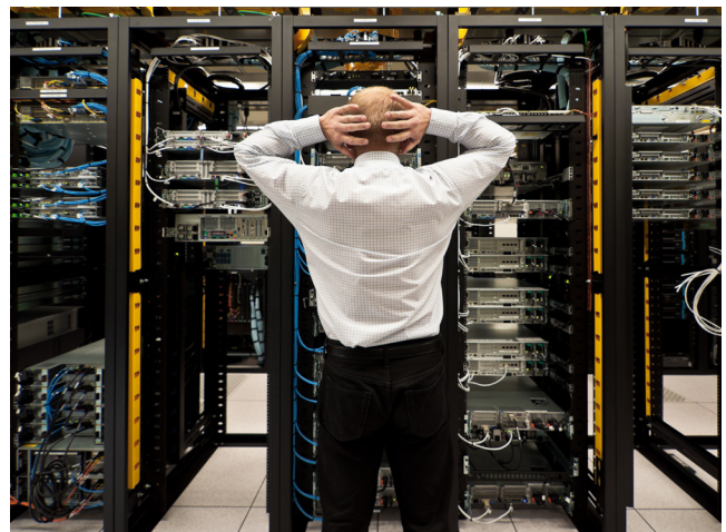
Air-cooled data centers are cold and noisy without the compute density of comparable immersion-cooling space.
